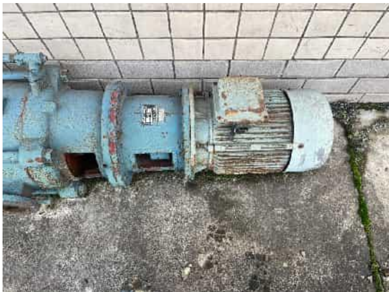
隧道机电设备7-8 -多级离心泵 (4)
